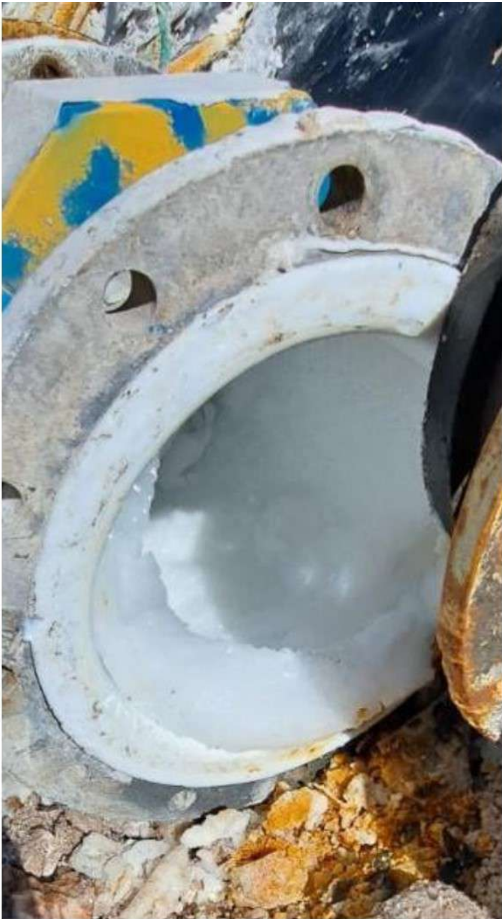
Incrustation in components (Flowmeter)
