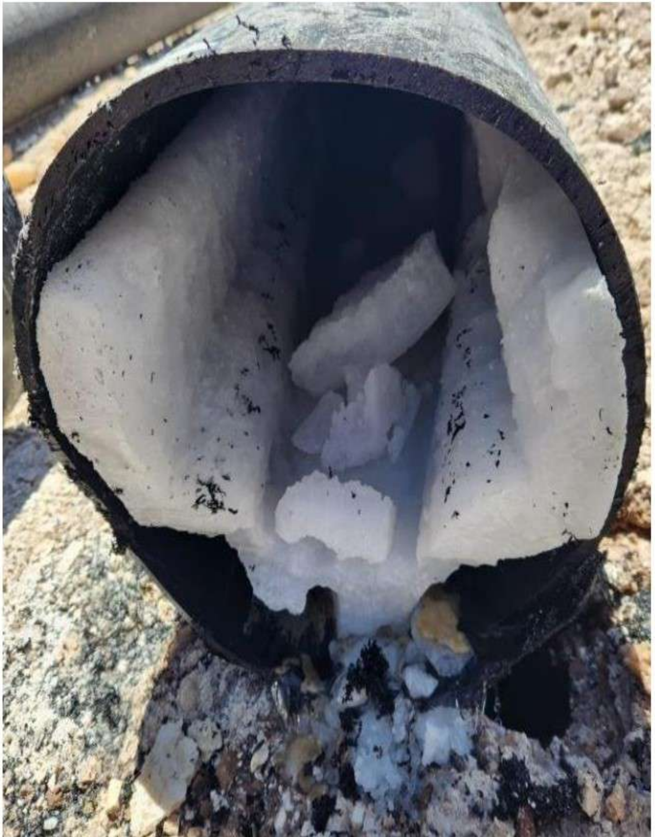
HDPE pipe inner incrustations
