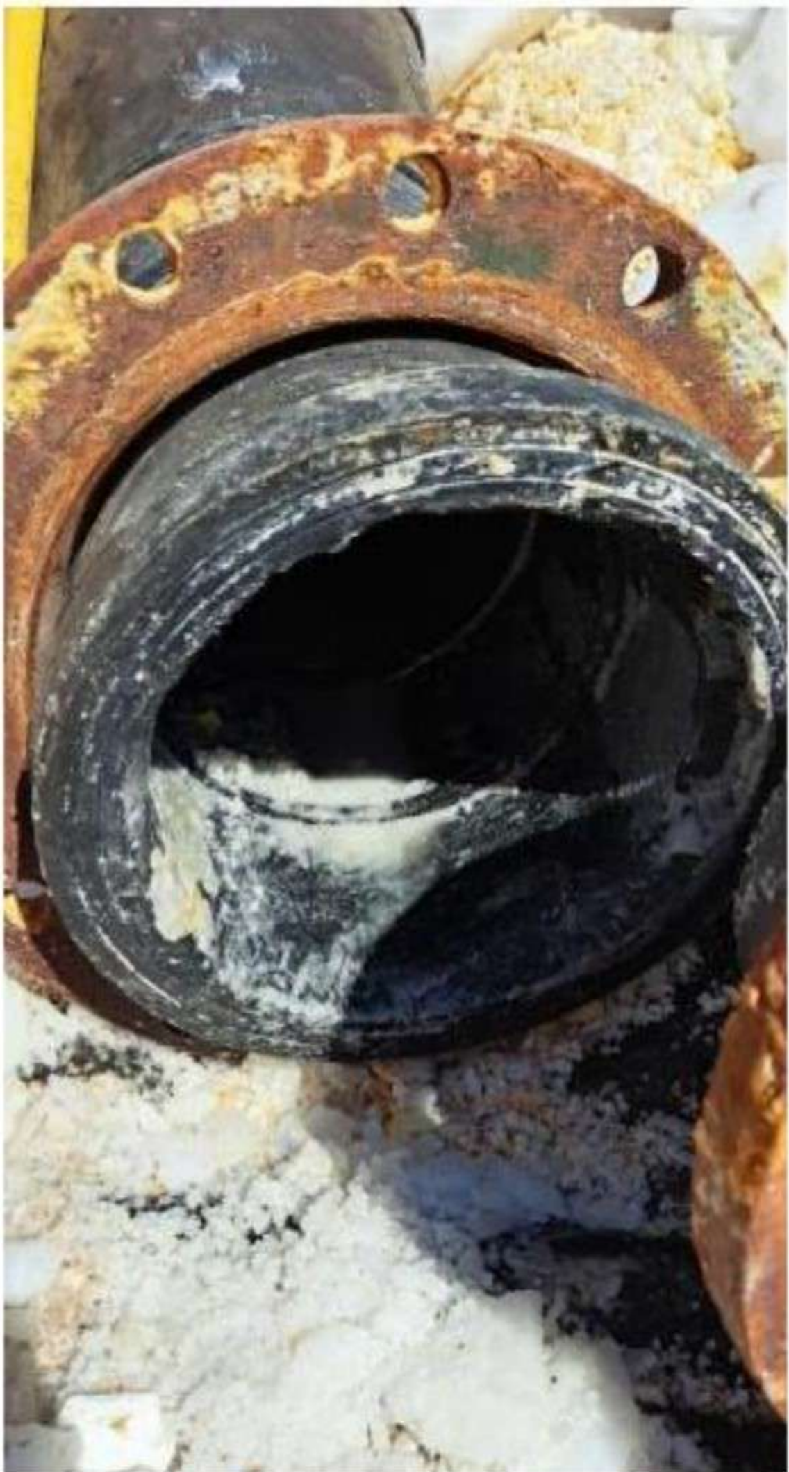
Incrustation in components (Flowmeter)
