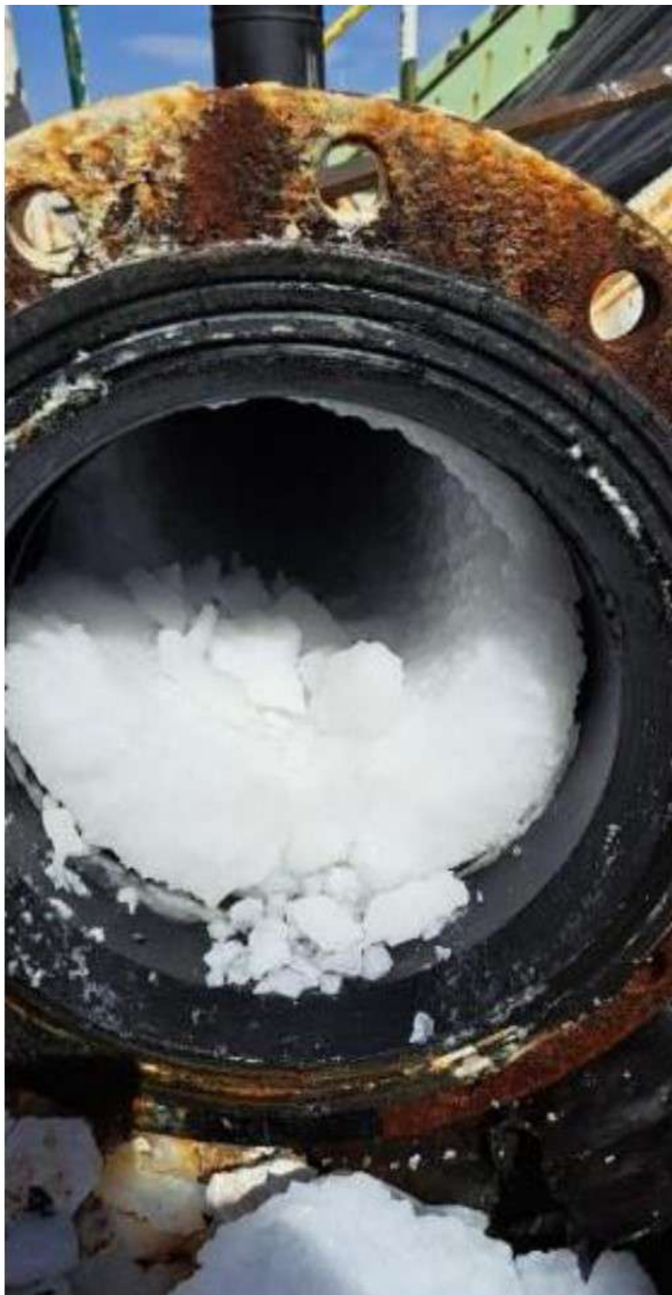
Incrustation in components (pump HDPE pipes before reaching the flowmeter - frequent incrustation sector)
